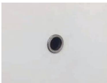
Hole within panel
