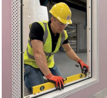
Adjust the position of the frame using the jacking screws to ensure it is aligned vertically and horizontally within the structural opening.
